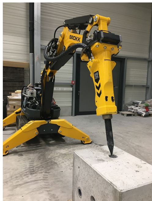
Fig. 1 The teleoperated demolition machine BROKK 170 and the experimental setup used in this work
