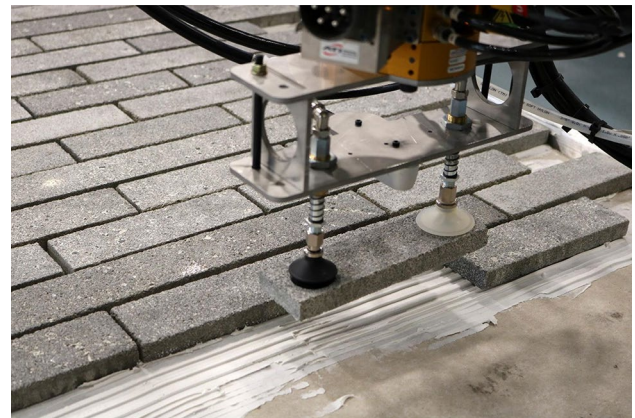
Fig. 6 Placing a cladding module in the assembly. Placement targets are calculated on the fly based on the assembly progress thus far and the dimensions of the material in hand
