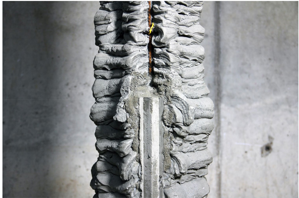
Fig. 15 A test that demonstrated how the vertical rebar can be encased in concrete after the concrete has set
