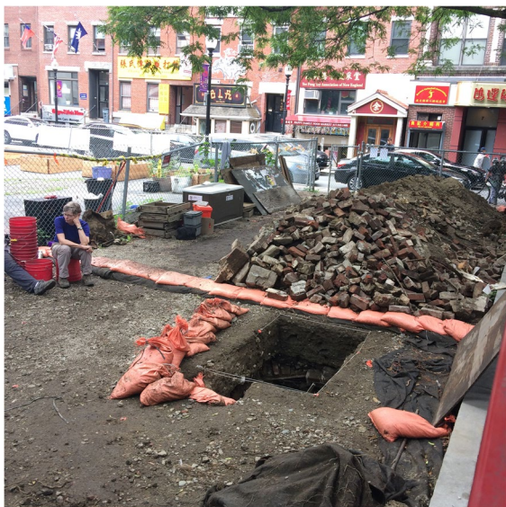
Fig. 5 View west across Trench 1 showing the extensive backdirt pile from the site trenches and nearby Chinatown businesses along Hudson Street in 2019. The individual row buildings seen in the background would have been nearly identical to the building located inside the project area. (Photo by Joseph Bagley, 2019.)
