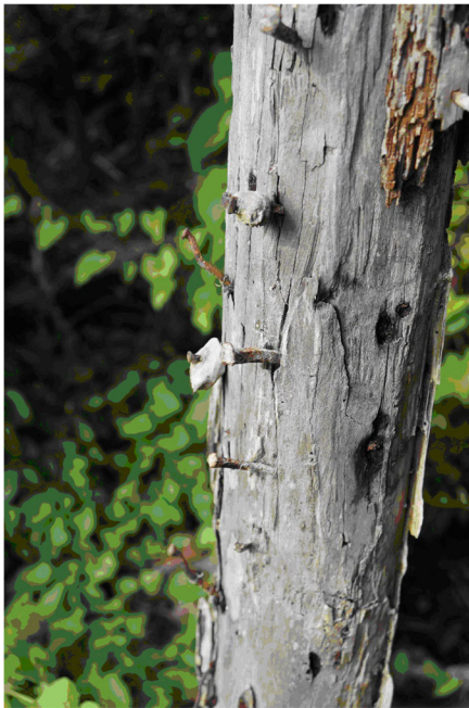
Fig. 5 Interior support beam from a mid-20th-century house in Crispeen, Saba, showing wrought, cut, and wire nails. (Photo by author, 2017.)
