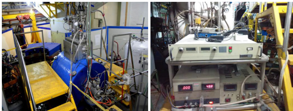
Fig. 1 (Color online) General view of the high-voltage platform installations
