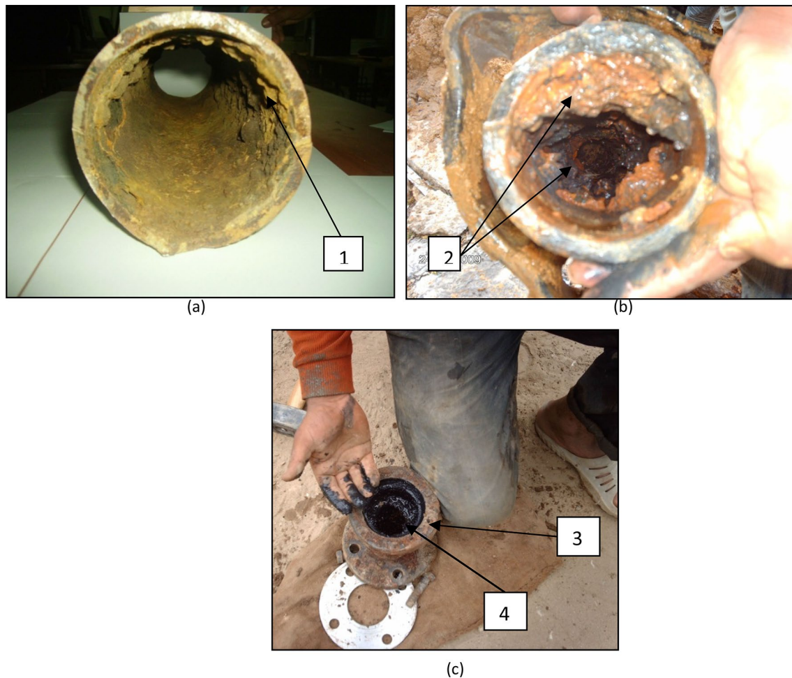
Fig. 4 Internal corrosion and contamination of cast iron water mains in the Faubourg neighborhood: a an old water main encrusted with deposits; b an old, heavily corroded pipe; c a flange containing dark mud (1 deposits, 2 buildup of corrosion, 3 flange, 4 black mud)
