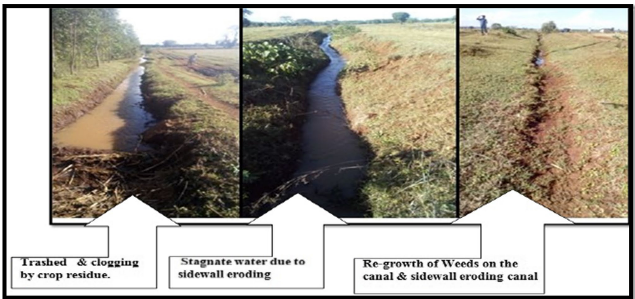
Fig. 7 Poor canal maintenance (unclean canals)
