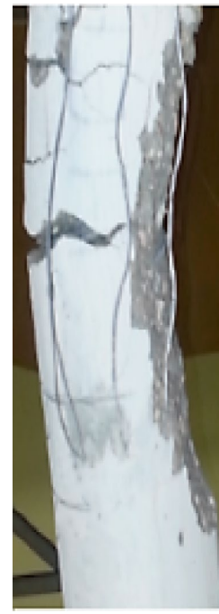
(c) Vertical cracks in upper and lower regions and horizontal cracks at mid-height [51]
