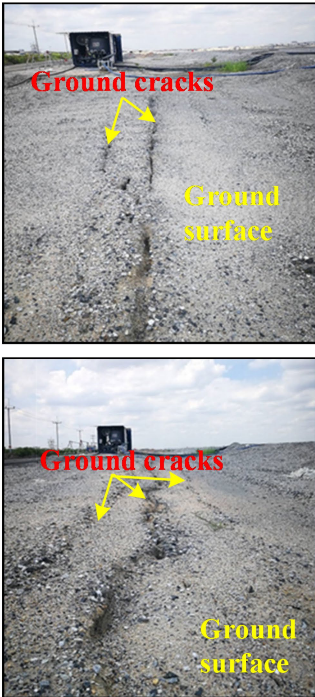
Fig. 13 Ground cracks due to vacuum pressure
