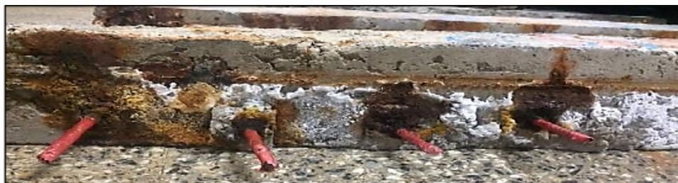
Fig. 6 Corroded beam specimen
