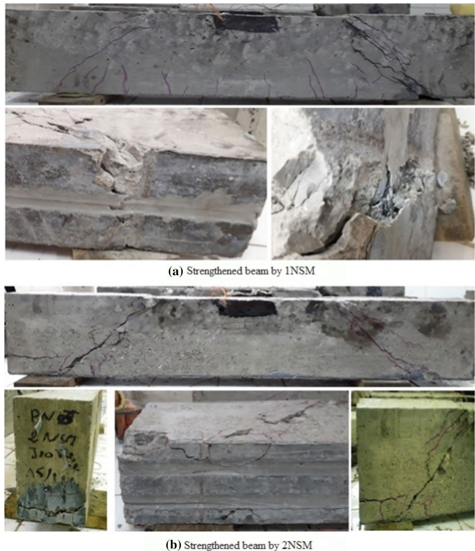
Fig. 7 Failure mode of strengthened beams by NSM technique
