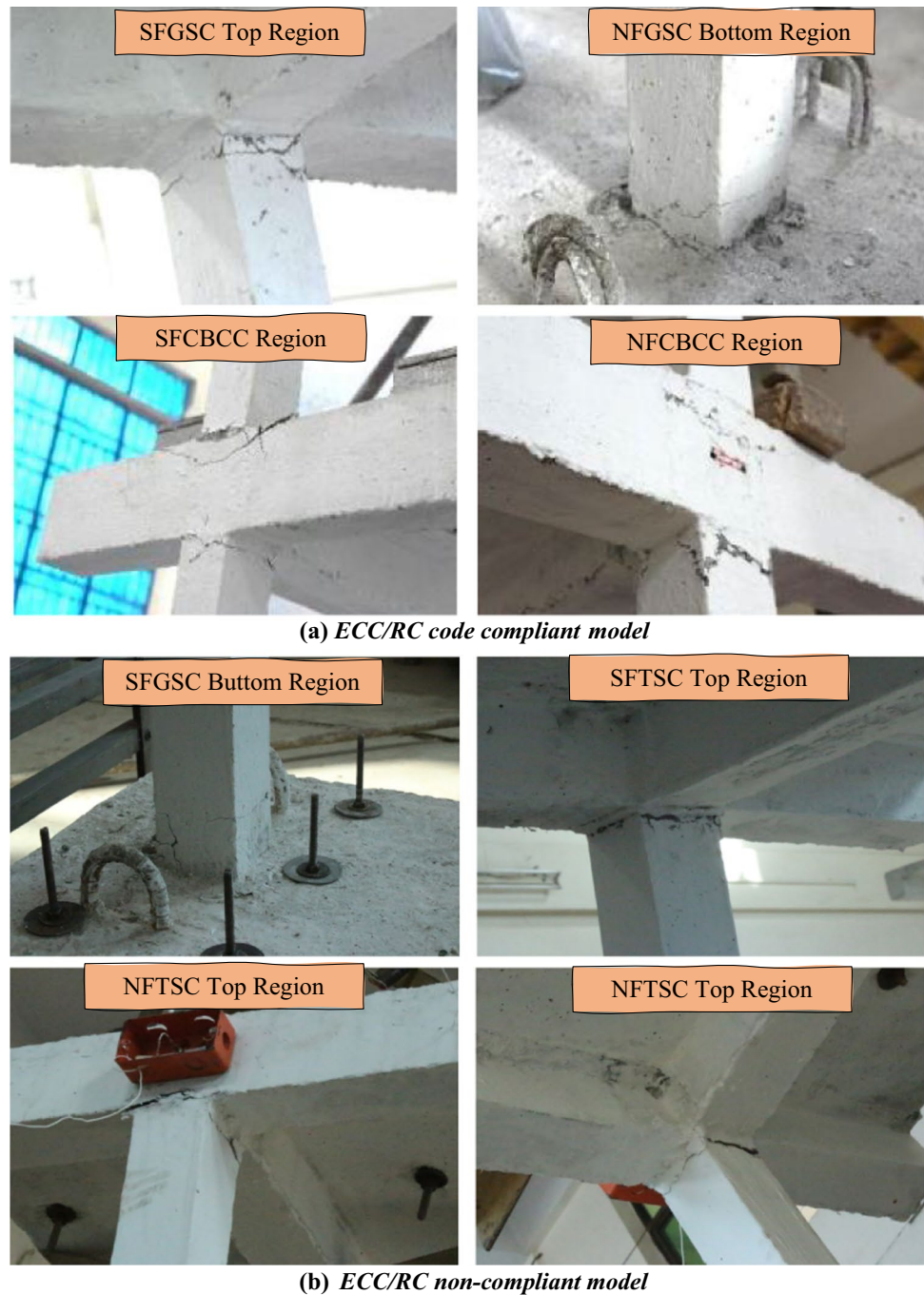
Fig. 7 Observed damages at the incipient collapse stage, Refer to Table 3 for damages evaluation
