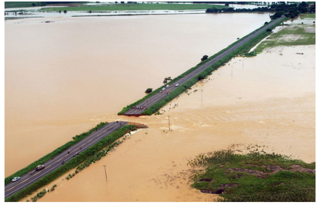
Fig. 2 Failure of Campos’s dos Goytacazes dam [6]
