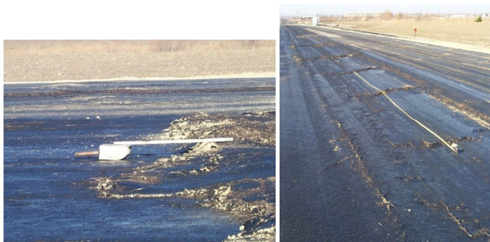
Fig. 2 Sulfate-induced pavement failure along US 67, Texas
