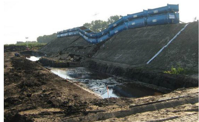
Fig. 6 Levee after failure [5]
