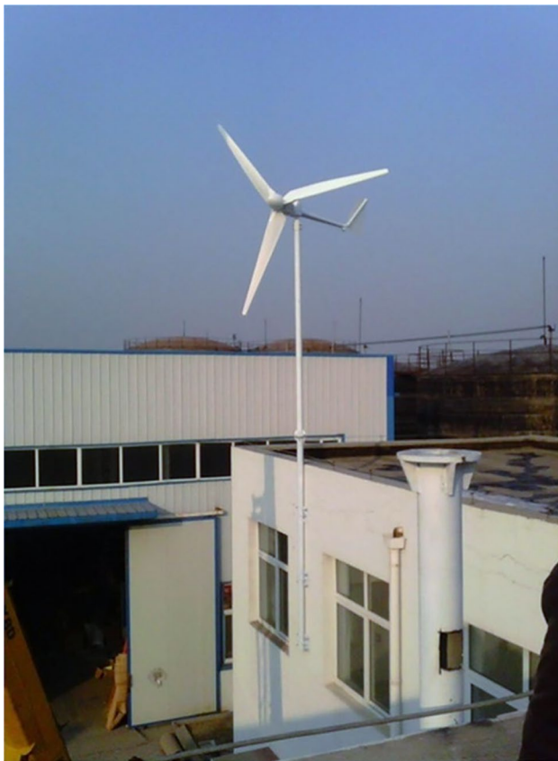
Fig. 8 HWT placed over the Rooftop (Pellegrini et al. 2021)
