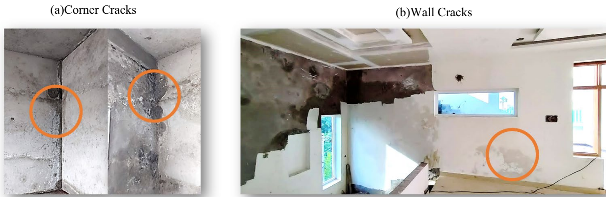
Fig. 1 Structural cracks in the concrete components of the building
