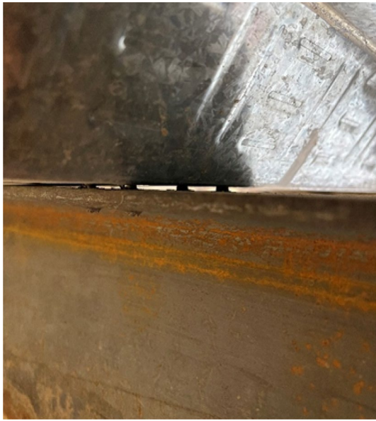
Fig. 24 Shear connector failure
