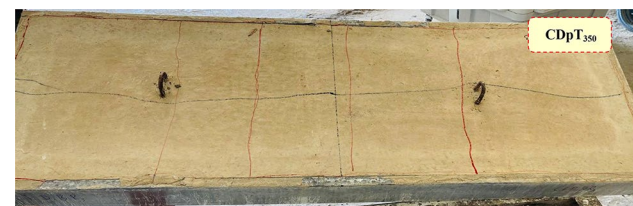
Fig. 21 Thermal and longitudinal cracking in specimen CD1T350
