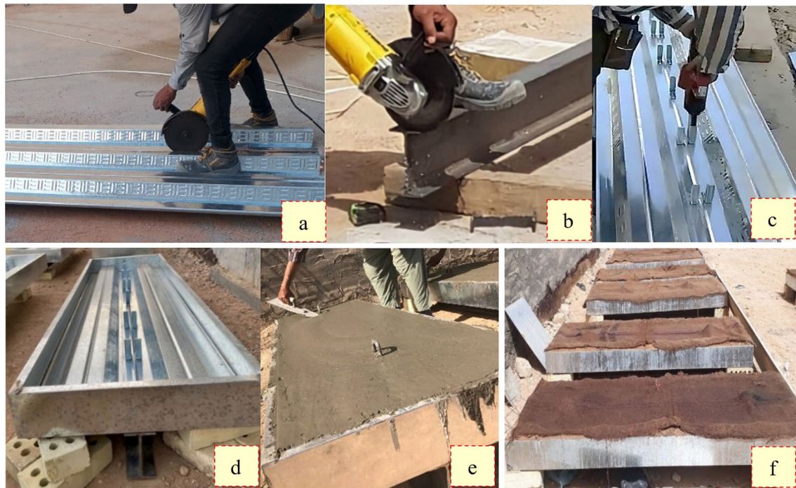
Fig. 4 The fabrication steps for composite beam specimens: a preparation of profiled steel plate, b ipe160 steel section preparation, c x-hvb shear connector positioning, d mold preparation for casting, e concreting f curing of cast specimens
