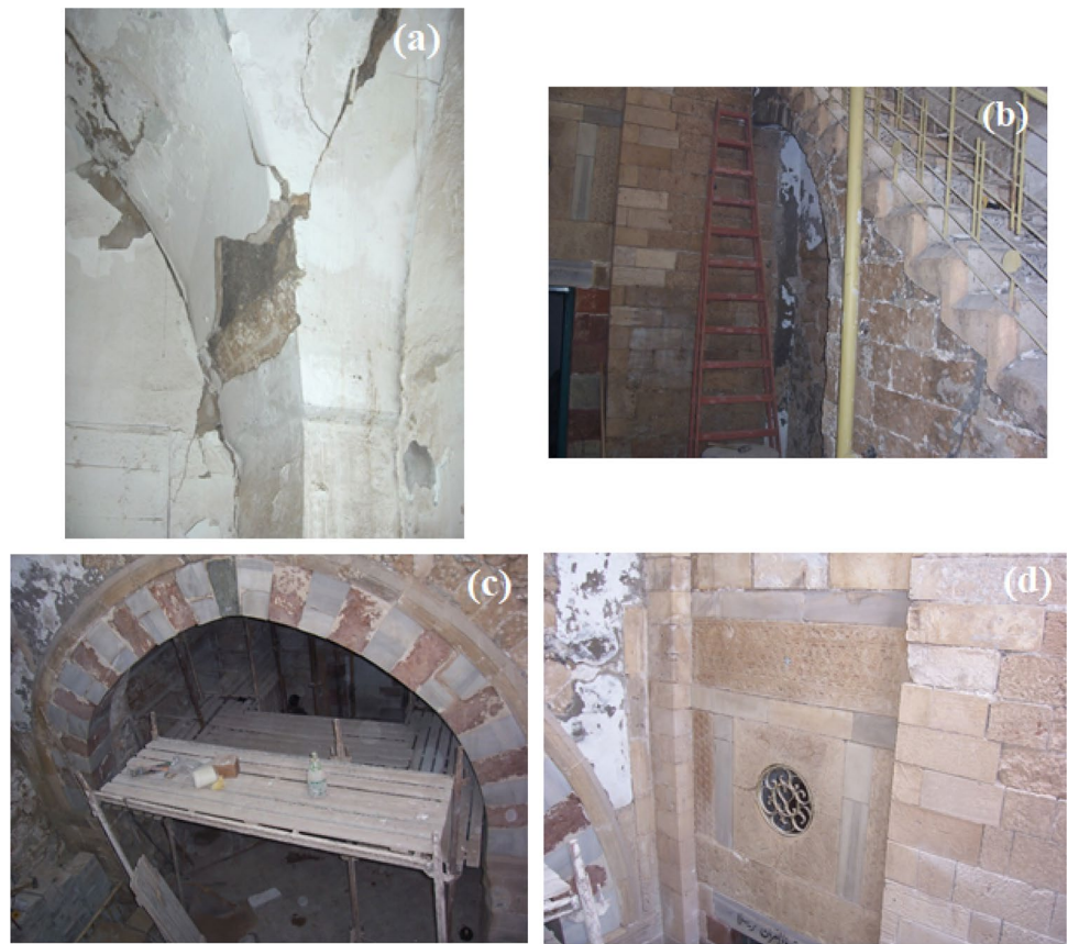
Fig. 2 Photos from Al-Ashi building. a Surface wear of the inner lining. b Internal staircase to access the second floor. c Platform for collecting samples. d Detail of the external coating of the building. Source: Archive of Islamic University of Gaza
