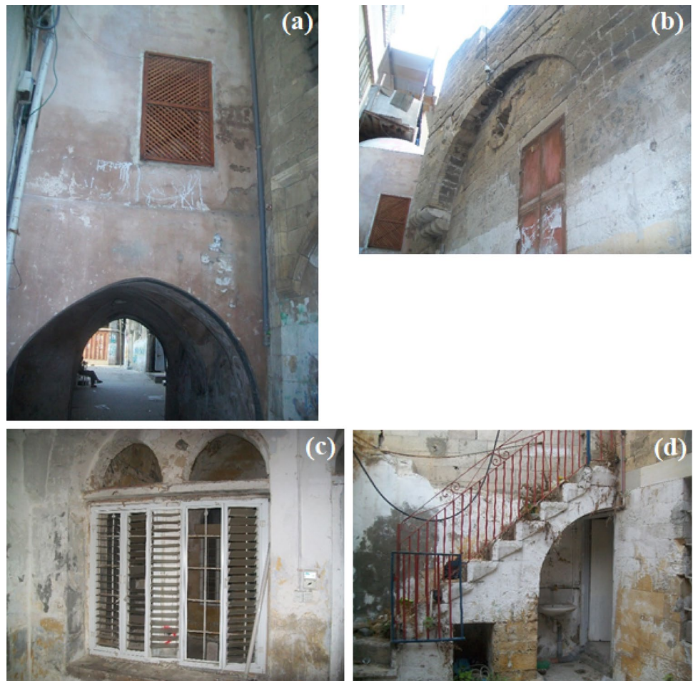
Fig. 4 Photos from Al-Hato building. a Arches of the external facade of the building. b View of the external facade of the building. c Detail of the degradation of the facade and windows. d Detail of the degradation of the external facade and access stairs to the second floor. Source: Archive of Islamic University of Gaza
