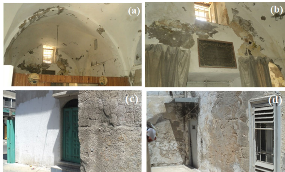
Fig. 3 Photos from Al-Ghussain building. a Degradation of the building internal roof. b Degradation of the building internal wall. c, d External coating of the building and details of degradation. Source: Archive of Islamic University of Gaza
