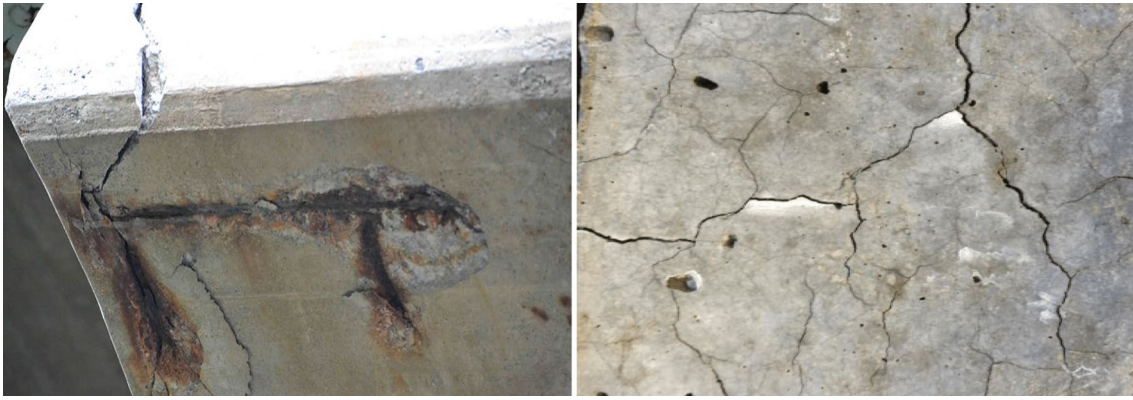
Fig. 15 Degradation of concrete structures from influence of aggressive chemicals
