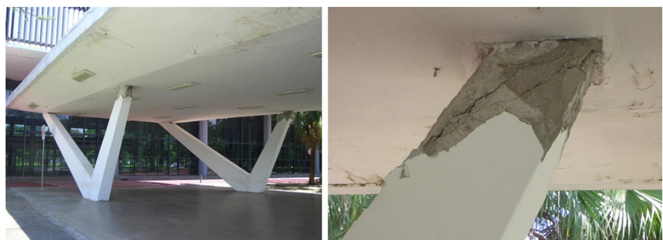
Fig. 15 End pillar of the marquee: a V-shaped geometry; b Cracking and partial rupture of the pillar head by thermal expansion of the slab
