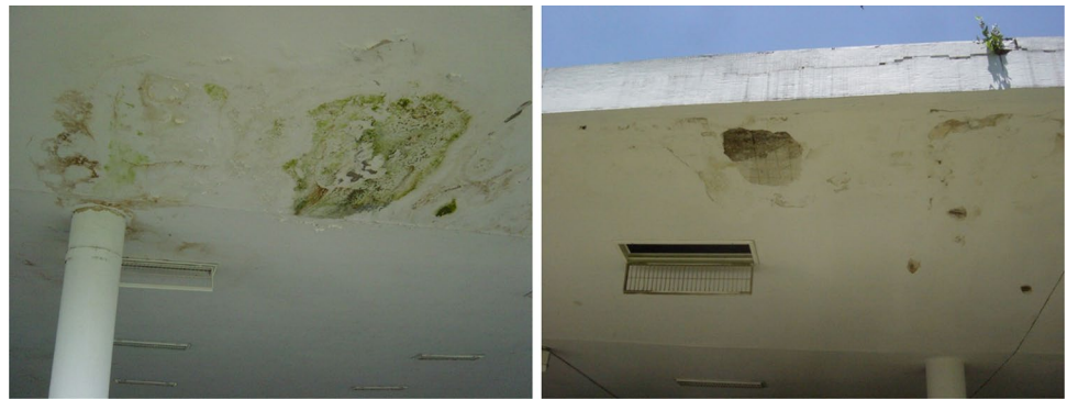
Fig. 18 Slab leakage deficiency, with rainwater infiltration and reinforcement corrosion
