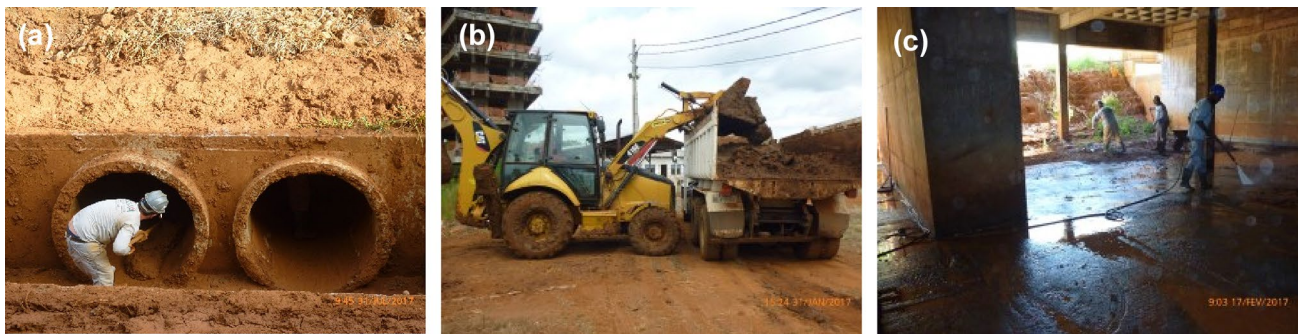
Fig. 11 a Cleaning services; b galleries mud removal; c main building underground cleaning
