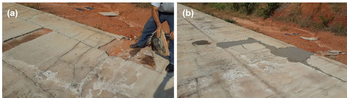
Fig. 12 a Removal of degraded waterproofing system; b correction of the same system
