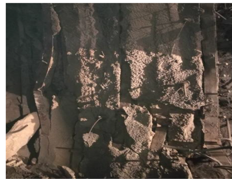
(b) torsion failure of double primary support
