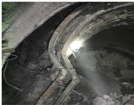
(a) crushing failure of double primary support
