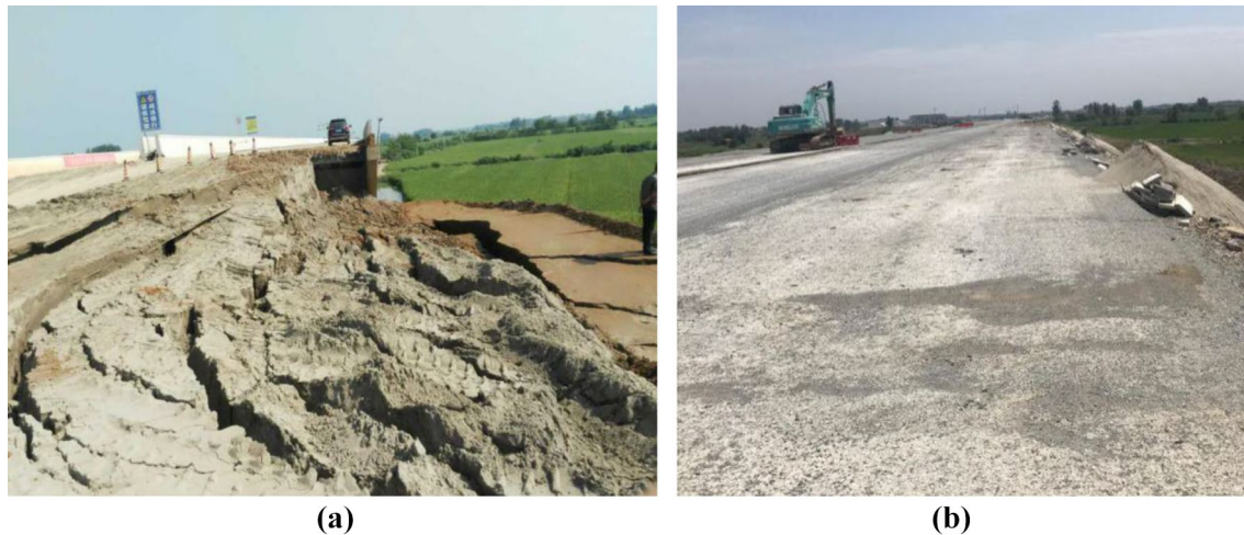
Fig. 3 a Failed highway embankment supported on floating piles; b completed highway embankment supported on end-bearing piles
