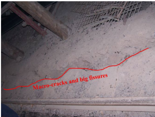
Fig. 31 Microfractures evolved into macrocracks or even big fissures on the roadway floor
