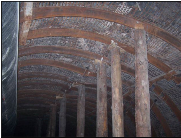
Fig. 29 The surrounding rocks are fractured and dilatant, finally producing heavy squeezing deformation
