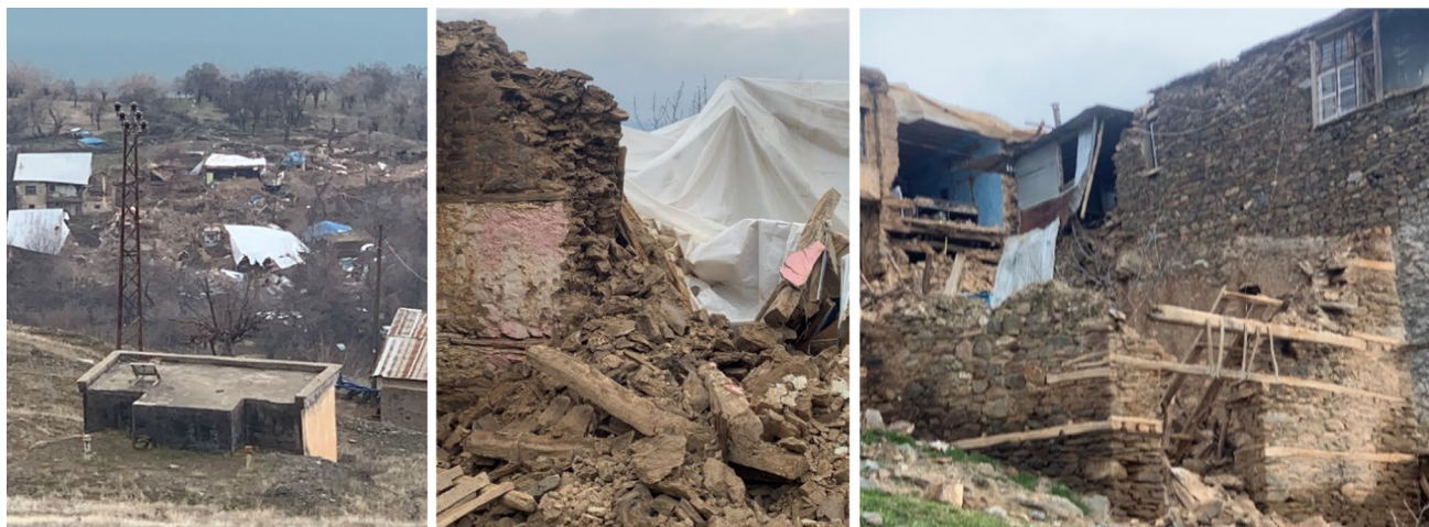
Fig. 10 Çevrimtaş village damages
