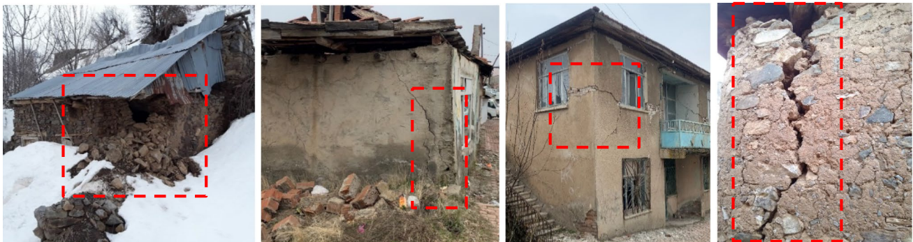
Fig. 18 Examples of corner damages
