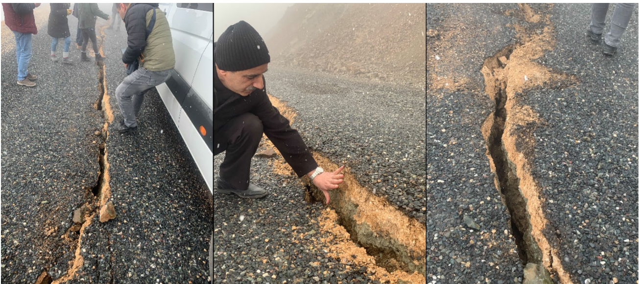
Fig. 9 Views of soil surface cracks on the highways by the earthquake (Çevrimtaş village, Sivrice)
