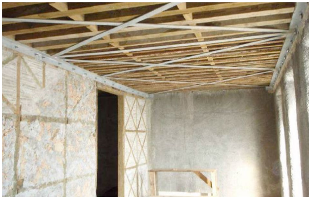
Fig. 26 Transversal anchorage system in multi-layer masonry walls (Adopted from Meireles and Bento 2013)
