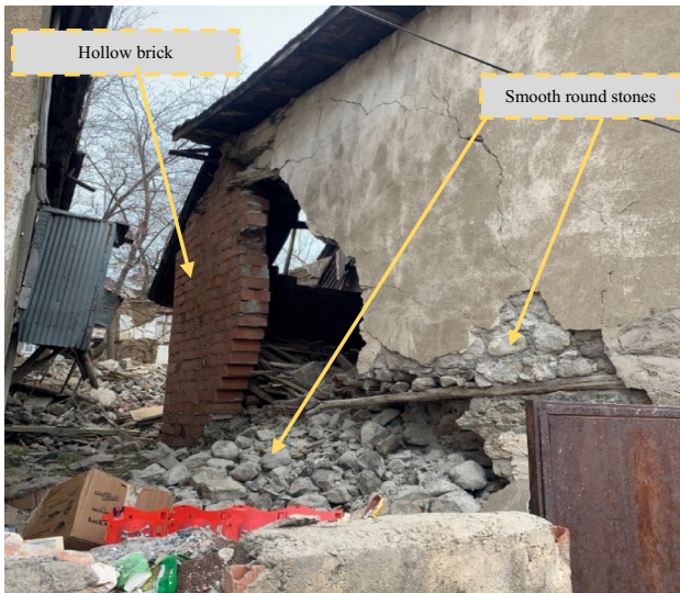
Fig. 12 Lack of horizontal and vertical bond beams and irregular use of different materials together
