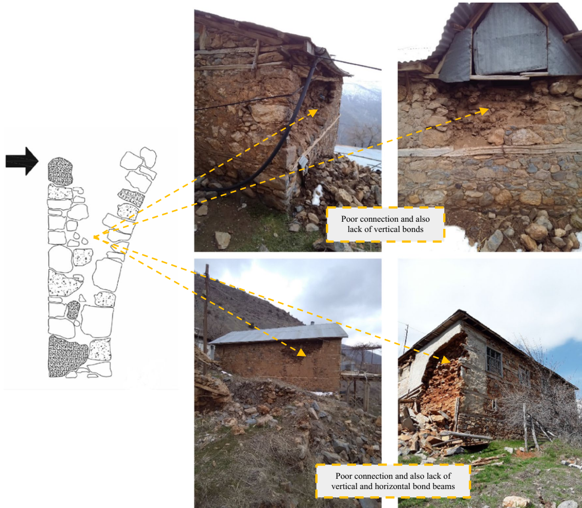
Fig. 20 Walls poorly constructed stone masonry building
