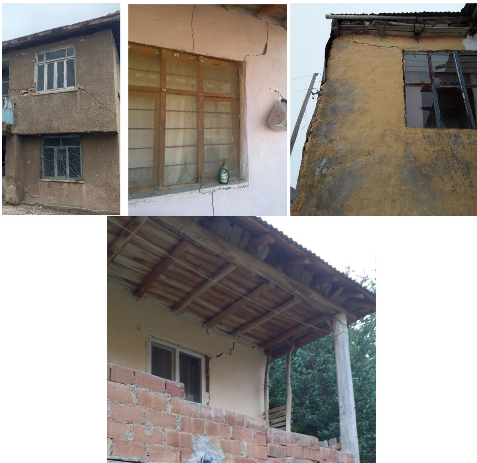
Fig. 15 Examples of cracks at corners of windows and doors of masonry buildings in Sivrice district
