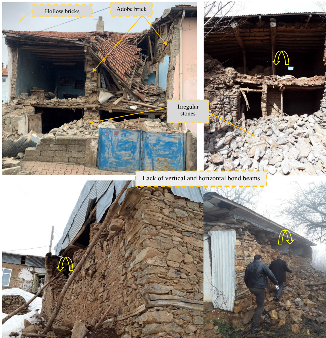
Fig. 11 View of out-of-plane failure on load-bearing walls
