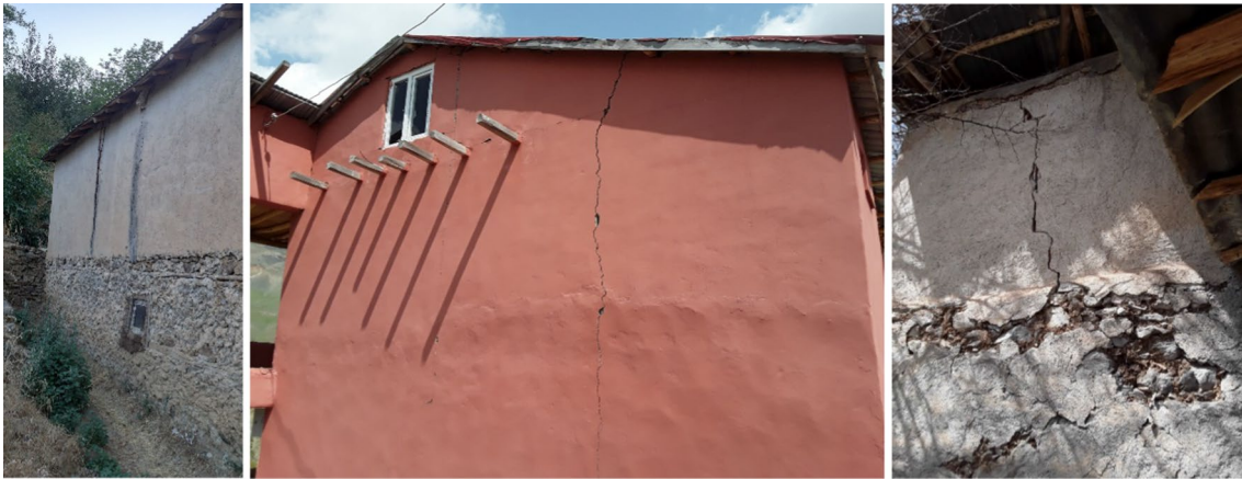
Fig. 17 Vertical cracks in low-strength masonry
