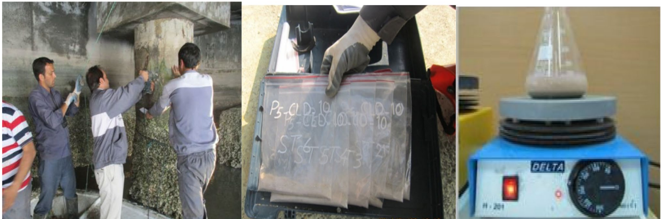
Fig. 10 Drilling of concrete piles and collecting powder from the restored concrete at wharf No. 5 in Imam Khomeini Port, Iran
