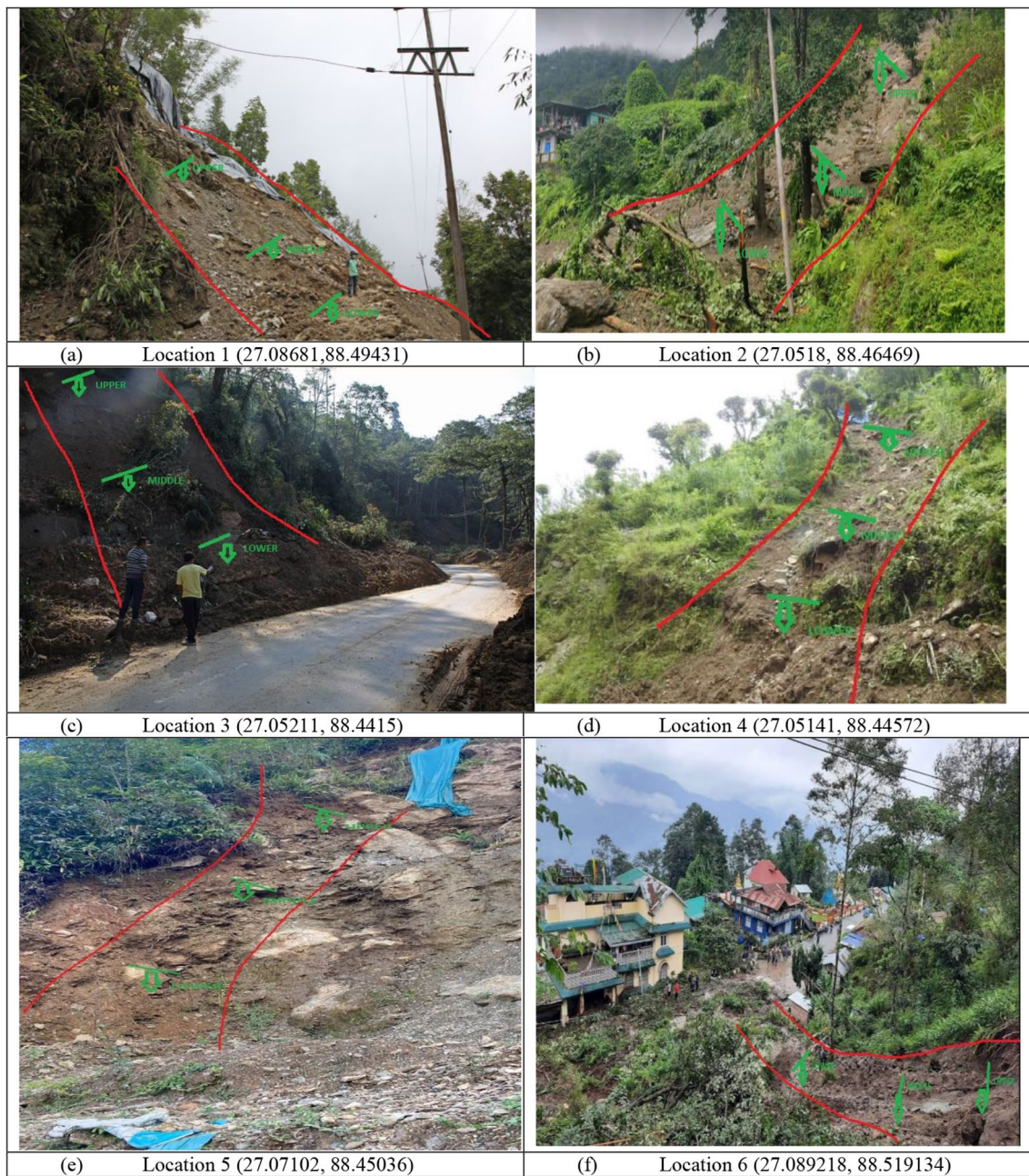
Fig. 2 Post-landslide images of critical locations
