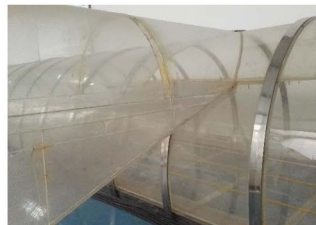
b Ventilation outlet
