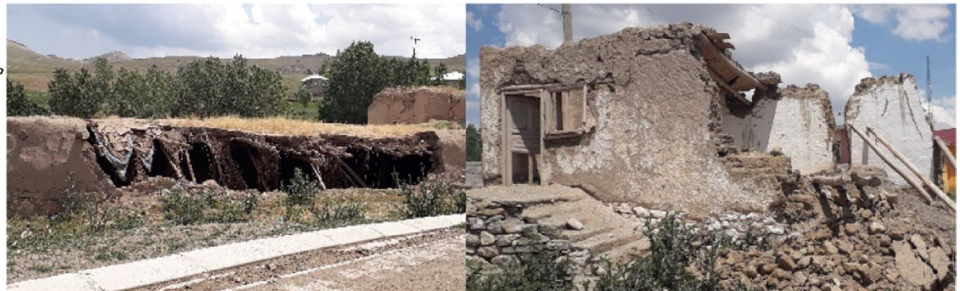
(a) Wall deformations caused from roof displacements
