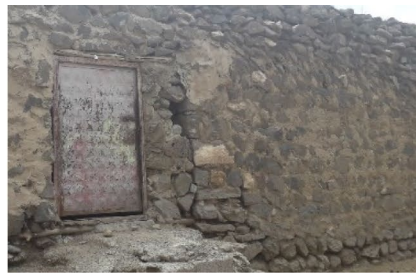
(e) Mixed style masonry wall (Ashlar corners, coursed base, coursed and random body, herringbone top)
