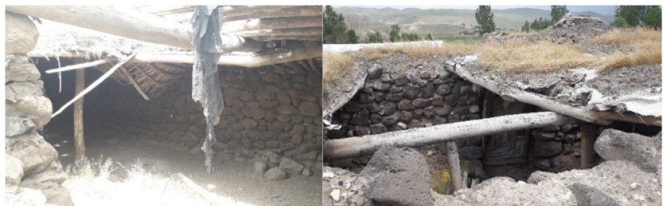
(b) Partial or total collapse of the roof
