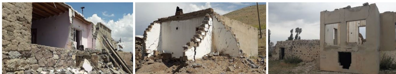
Fig. 20 Damaged newly constructed lightweight pumice block buildings
