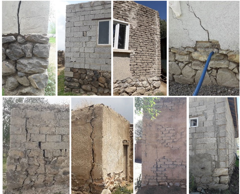
Fig. 12 Wall cracks due to the foundation movement during earthquake
