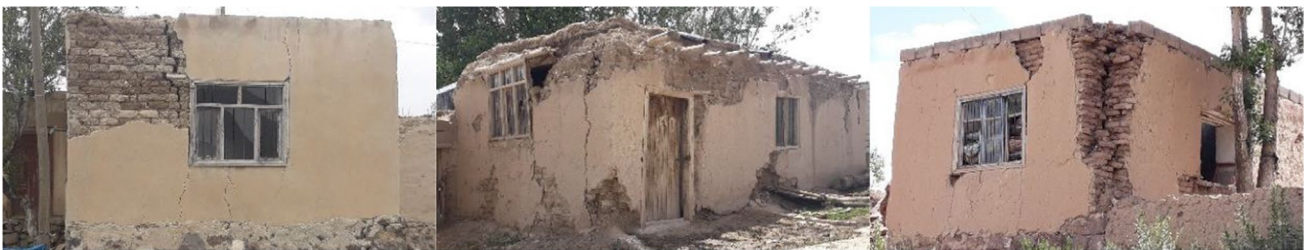
Fig. 17 Damage around openings
