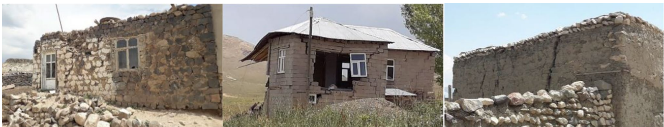
Fig. 18 In-plane damage in the walls
