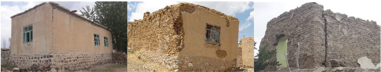
Fig. 16 Breakage of the link between the walls
