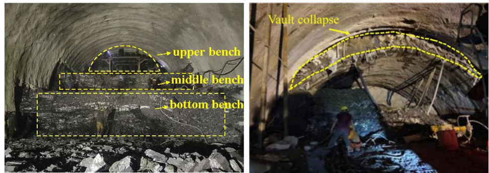
Fig. 2 Tunnel construction and vault collapse in the tunnel
