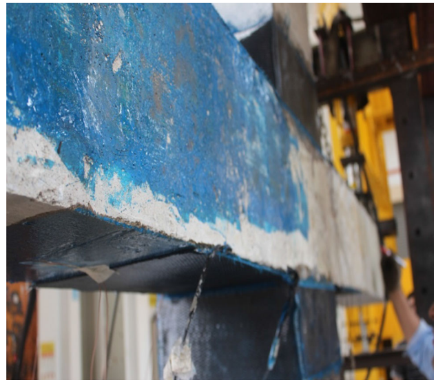
Fig. 4 Joint strengthened by CFRP wrap in columns region with L-shape overlays on the top and bottom of beams (Behind view)
