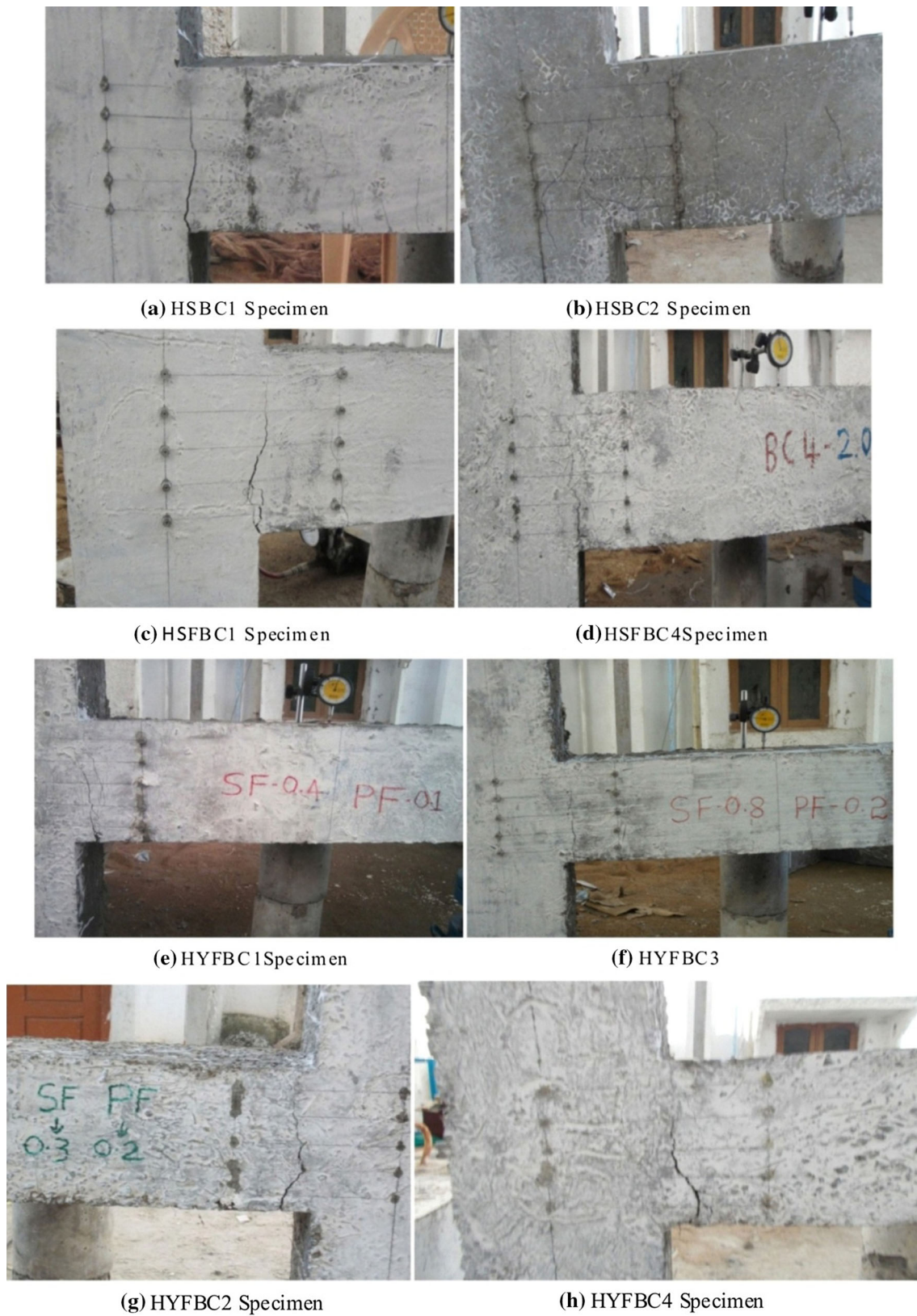
Fig. 11 Crack patterns of specimens after testing
