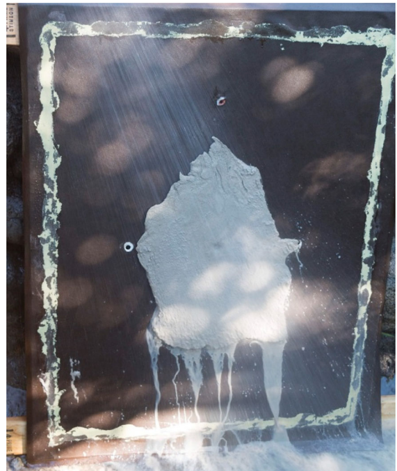
Fig. 7 The grouted island still attached to the separated wall
