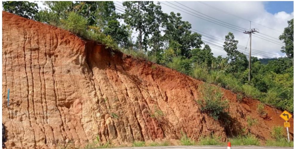
Fig. 1 Highly eroded back slope at Highway No. 1192, Chiang Mai Province, Thailand, where the soil sample was taken
