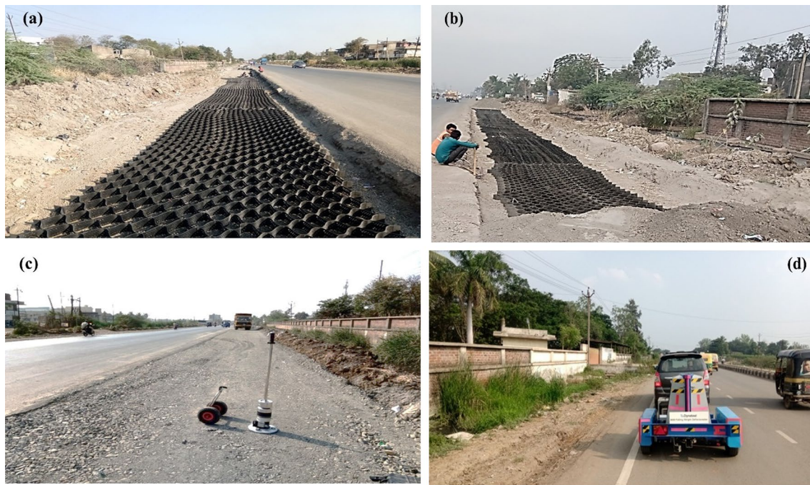
Fig. 2 a Installation of geocell, b filling of geocell, c LWD testing over the base layer, and d FWD testing over bituminous layer
