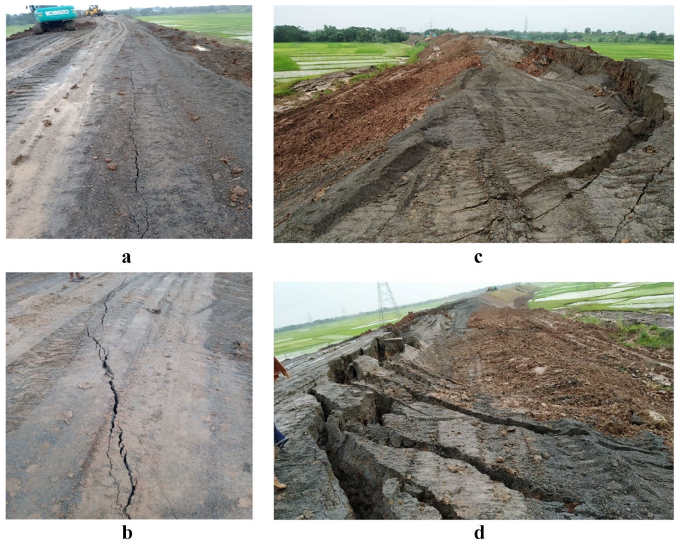
Fig. 2 a Development of the first crack on the formation. b Crack expansion and propagation leading to slope failure. c Observance of deep vertical cut on the post-failed embankment. d Failed and intact embankment along the curved alignment
