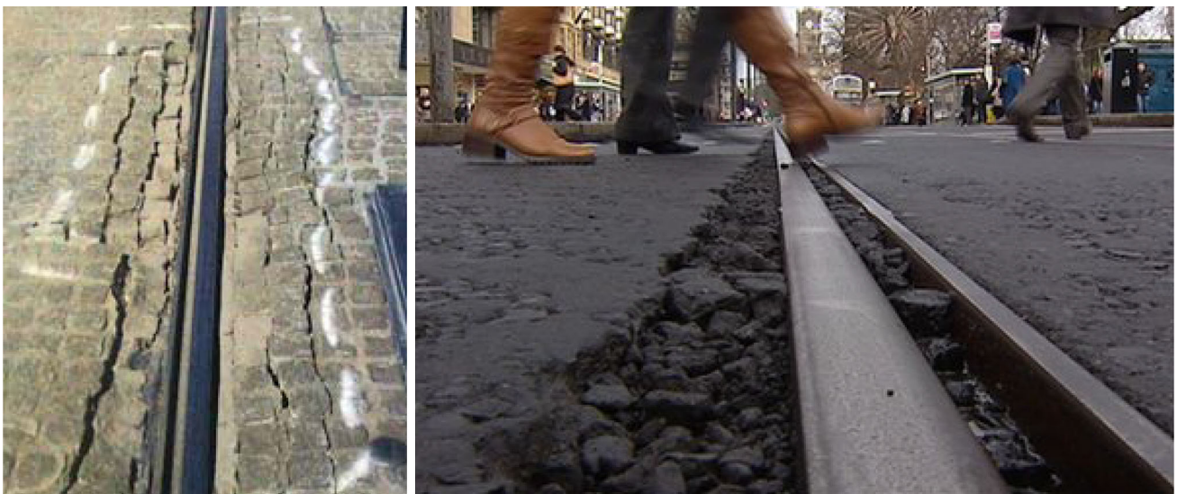
Fig. 11 Damages to road and tramway superstructures [20]
