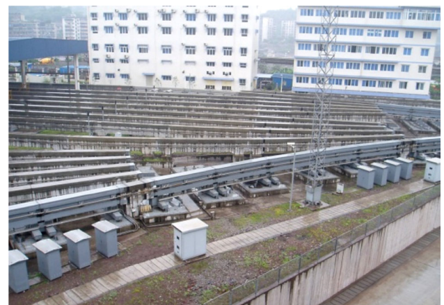
Fig. 7 Switch area of line 2 depot in Chongqing
