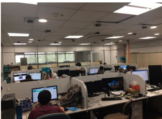
Fig. 14 Smart lighting system installed in researcher room 3 with daylight harvesting
