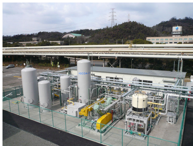
Fig. 14 3 tons/d pilot scale PSA facility
