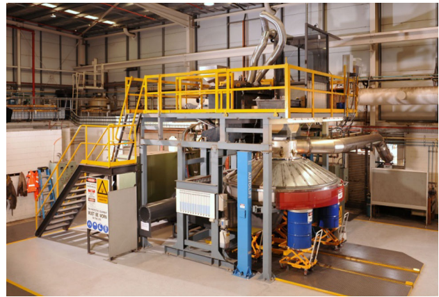
Fig. 13 The semi-industrial scale (3 m in diameter) integrated heat recovery and dry granulation pilot plant at CSIRO with design throughput of 6 t/h of slag [52]
