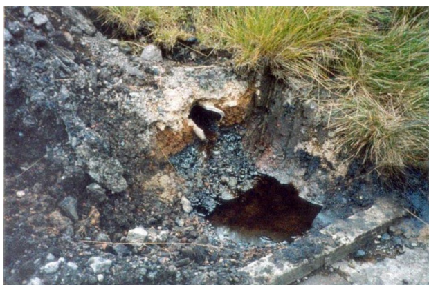
Fig. 1 Coal tar NAPL leaking from a broken pipe in a former coking works
