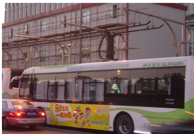
Fig. 24 Supercapacitor bus at the charging station also used as a bus stop
