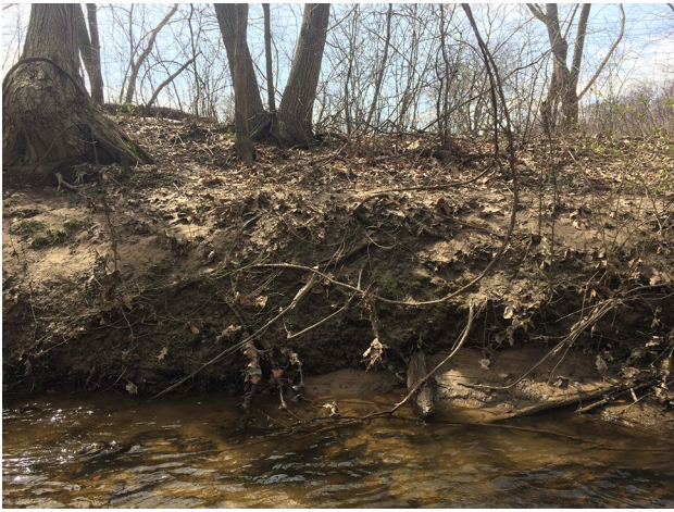
Fig. 14 Sandy eroding banks observed in subbasin B12 in the lower Indian Mill Creek watershed, April 2017
