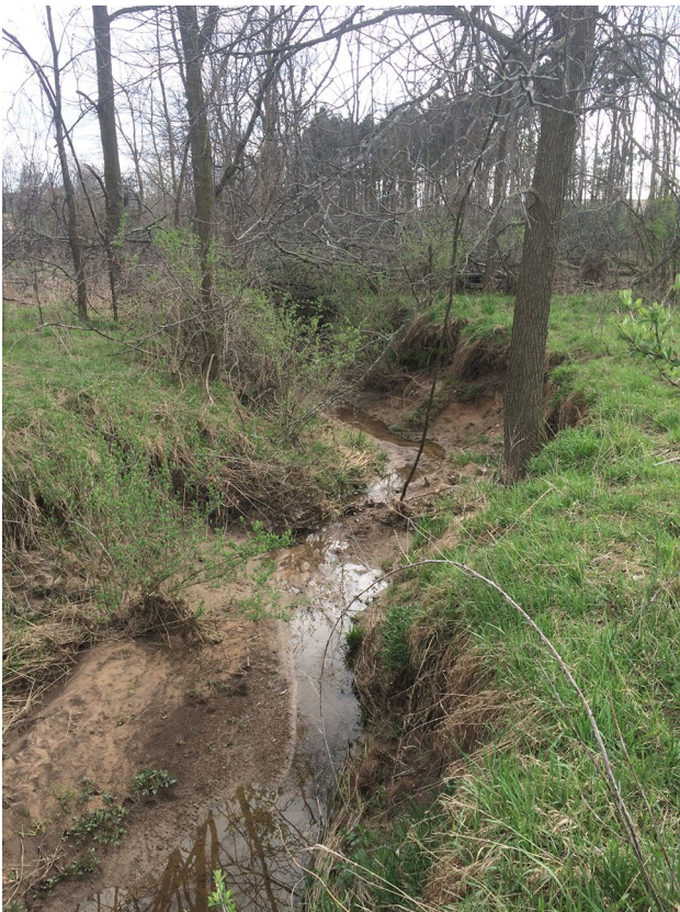
Fig. 15 Severe incising and bank erosion observed in Walker Avenue Ditch (subbasin B11) of the Indian Mill Creek watershed, April 2017
