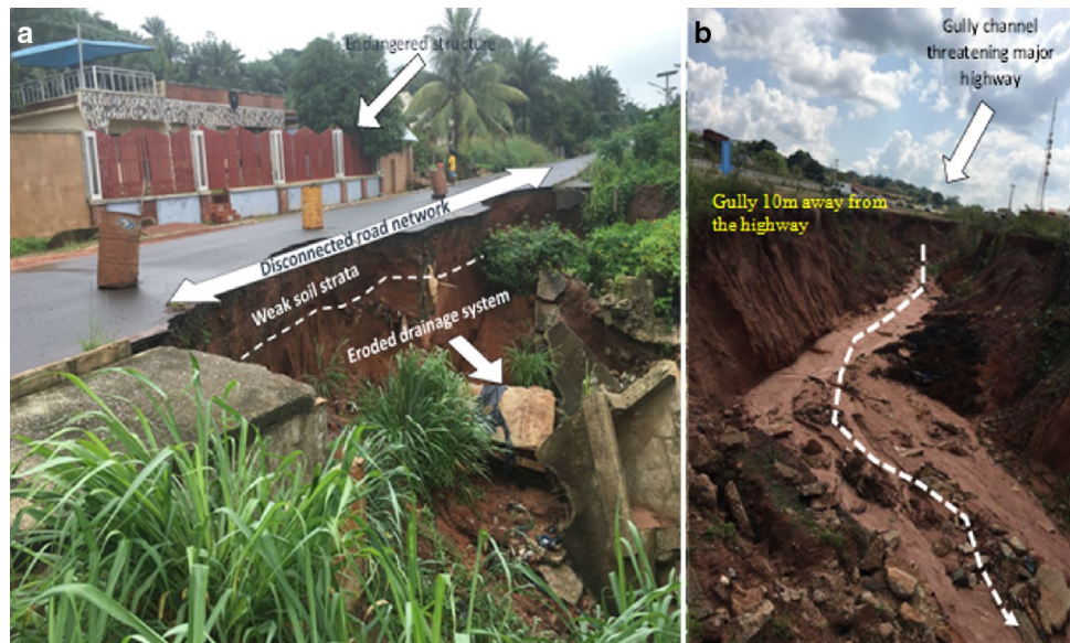
Fig. 1 a, b Developing gully channels destroying and threatening engineering structures in Udi province
