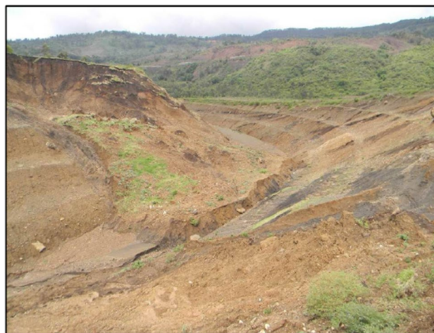
Fig. 3 Landslides triggered by construction of the section of road between Wozeka and Gedole
