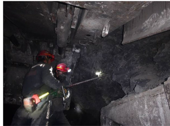
( b ) Roof caving accident
