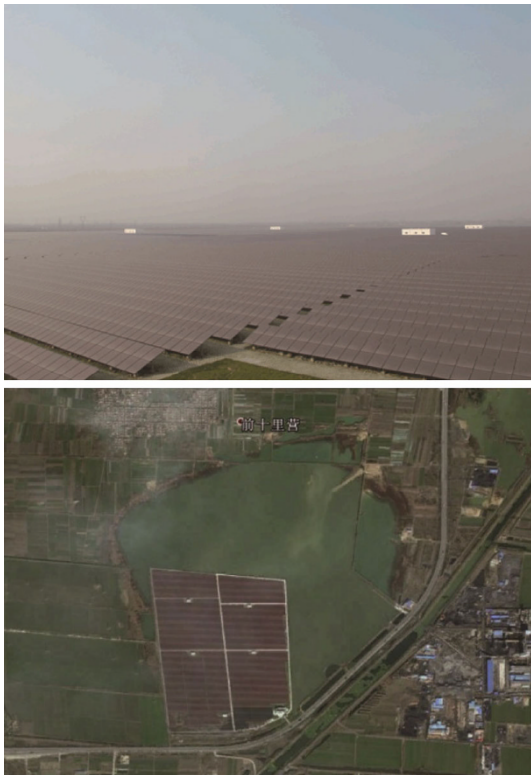
Fig. 4 Huahan solar photovoltaic power plant in southeast Jining city
